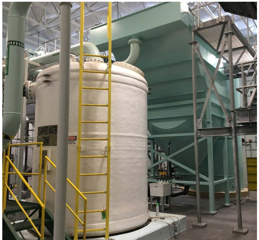
Parallel Plate Clarifier
